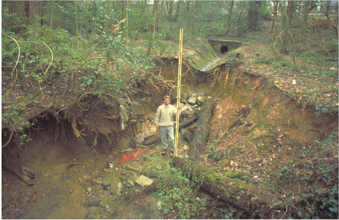
Figure 4: Stormwater Culvert Carrying Road Runoff Into the Head of the Stream Draining the Deepdene Watershed
