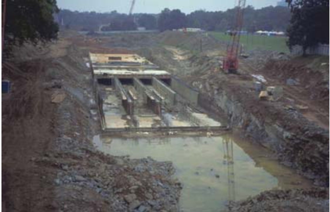
Figure 27: One of Atlanta's Stormwater Treatment Plants
